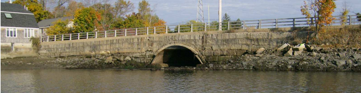
PHOTO 1 Overall view of culvert and wall looking north. Taken 10-21-09 by D. Mellor
