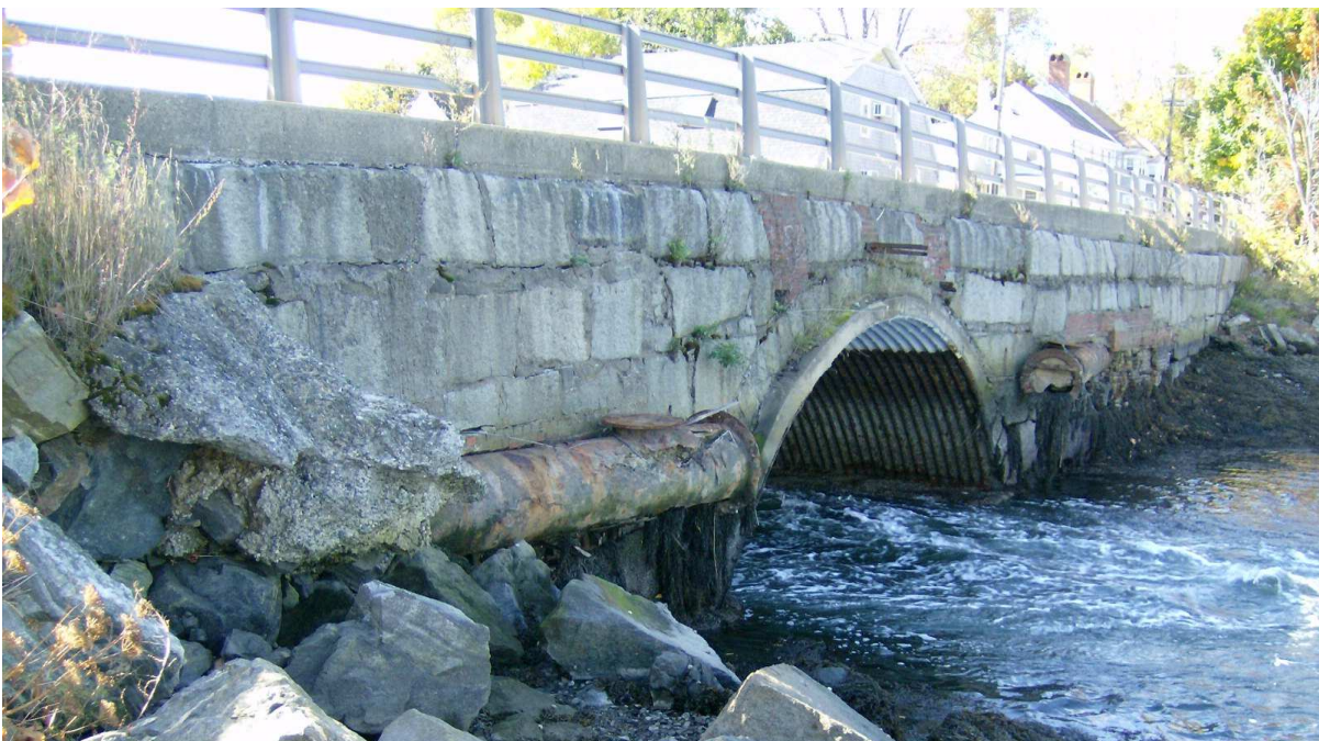
PHOTO 3 Wall and culvert looking southwest, note abandoned sewer line to be removed. Taken 10-14-09 by D. Mellor
