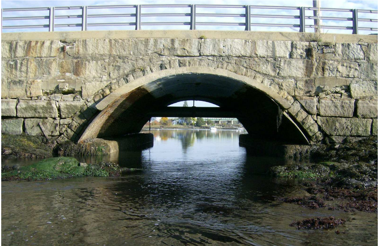
PHOTO 4 Culvert looking north, note sewer line to be moved. Taken 10-21-09 by D. Mellor
