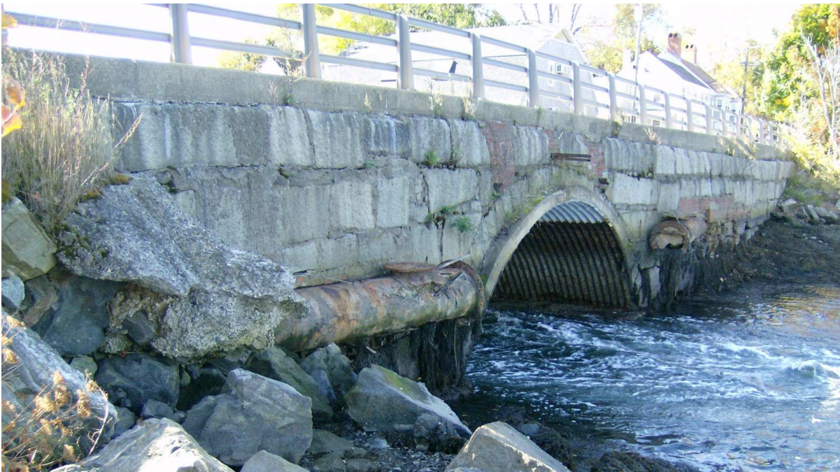
PHOTO 3 Wall and culvert looking southwest, note abandoned sewer line to be removed. Taken 10-14-09 by D. Mellor
